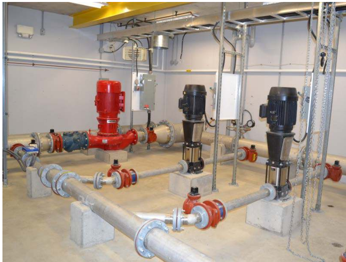
New Water Booster Station pumps.
